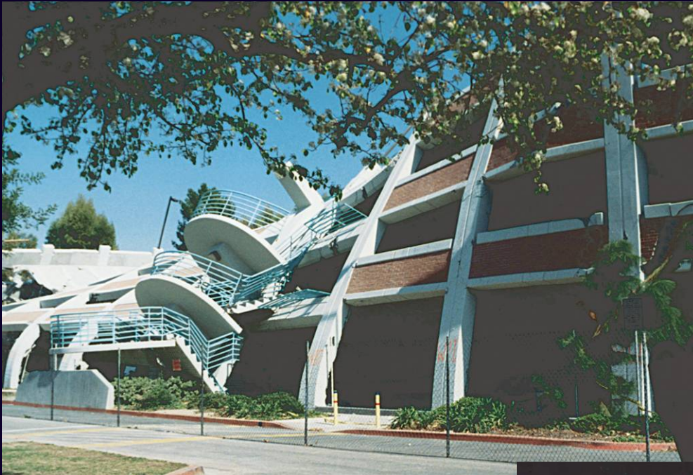
Parking Structure C: 1994 earthquake
